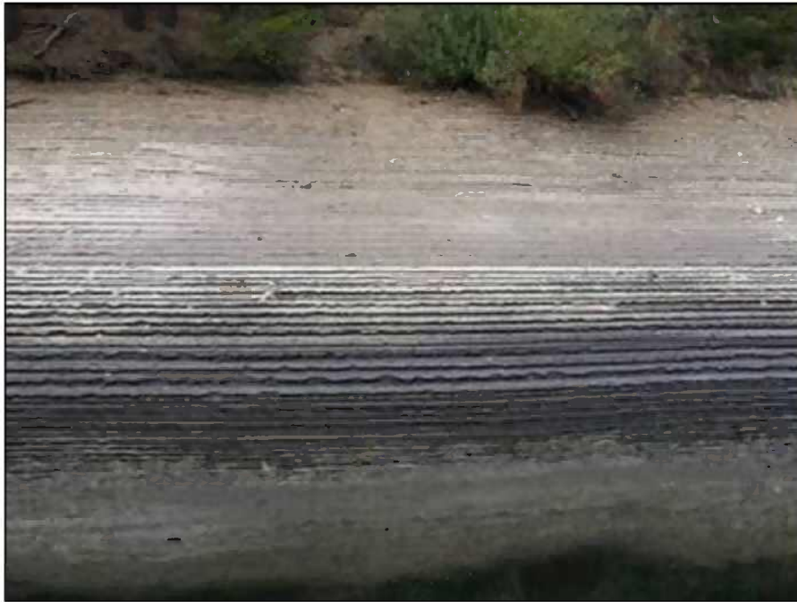
Figure 24. Erosional bands on the east shore of Reeder Reservoir created during drawdown. The light colored material in the middle is largely coarse sand comprised of “rotten” granite and the dark material is organic matter deposited during full-pool conditions. This image was taken on September 14, 2007, with the reservoir stage at 2851 ft (21 ft below full pool).
